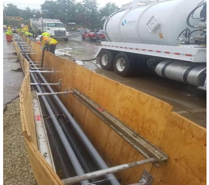
Fig 2: Vac truck is used to pump rain water out of trench in "A" lot. Viewing south. (6-20-19).
