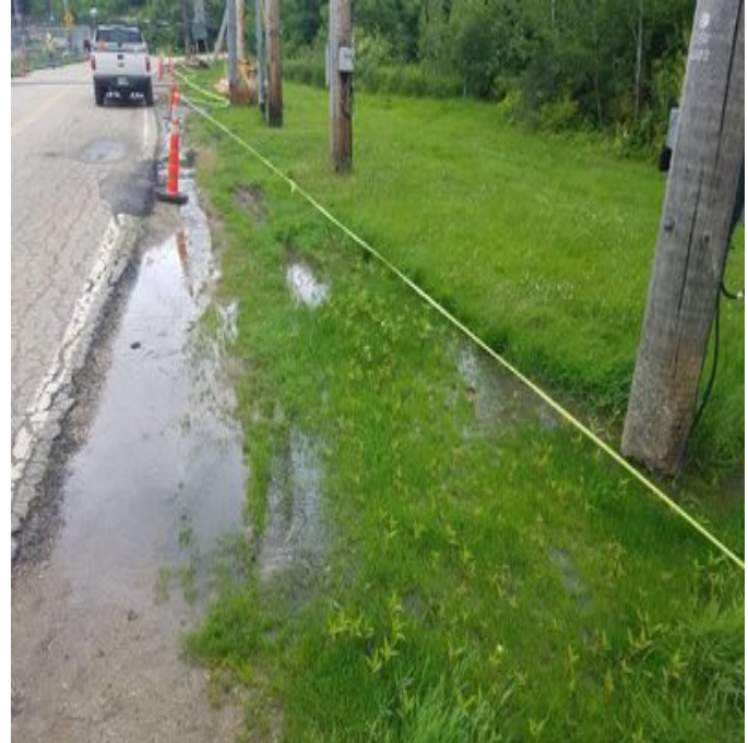
Fig 8: Filtered water flowing next to Colovos and back into grassy area north of College Brook. Viewing north. (6-21-19).
