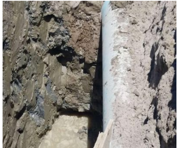
Fig 14: Residual water/rain water seeping out during excavation. Viewing north. (6-24-19).
