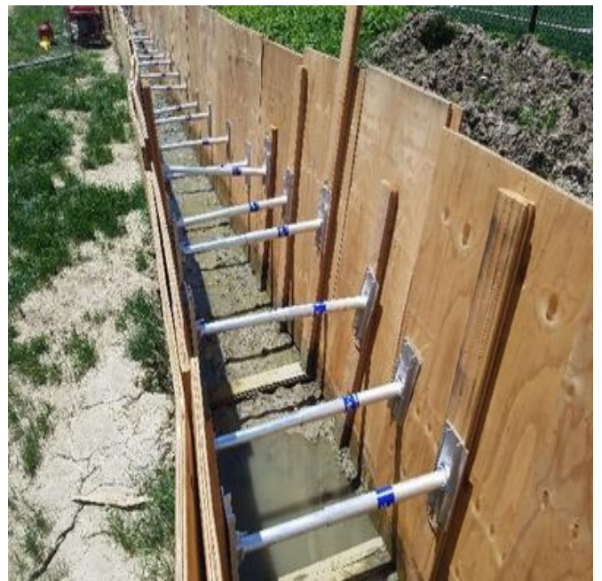
Fig 12: About half of the water in the trench along Colovos Rd has been pumped out. Viewing south. (6-24-19).
