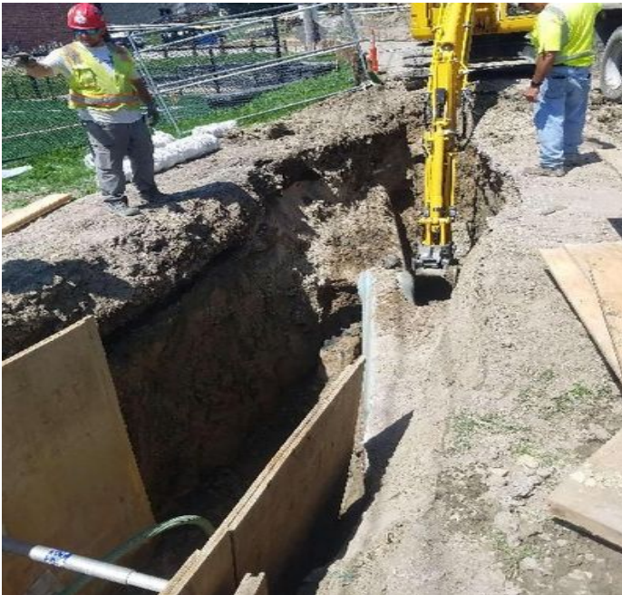
Fig 15: McCourt uncovered an old asbestos water line during excavation. Viewing north. (6-24-19).
