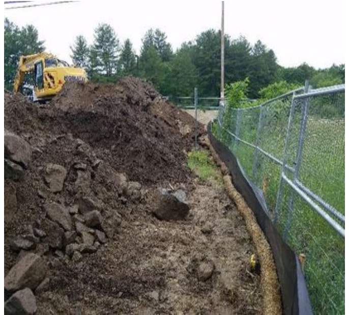
Fig 26: Silt fence and straw wattle installed between Waterworks Rd laydown yard and wetland DW65. Viewing west. (6-26-19).
