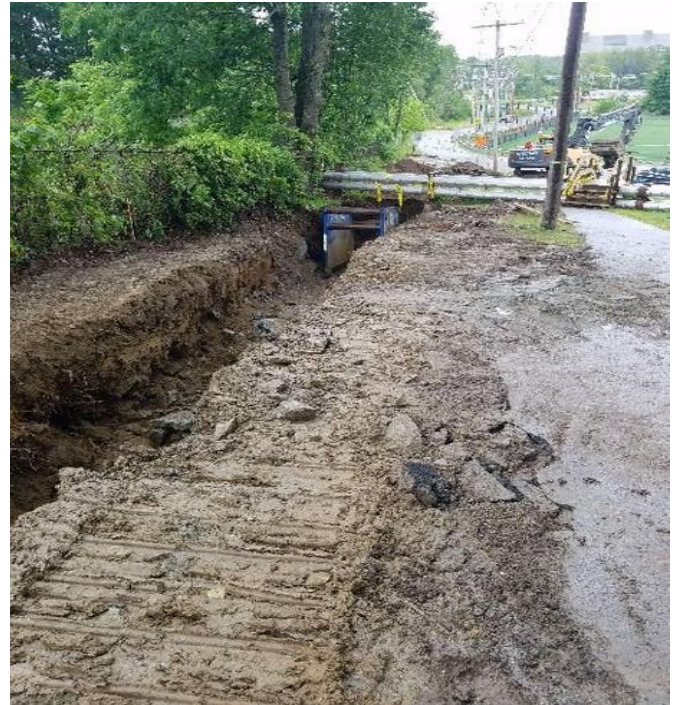
Fig 4: Trenching for duct bank next to field house at UNH. Viewing south. (6-21-19).
