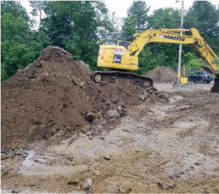
Fig 25: Soil stockpiled in the Waterworks Rd laydown yard continue to be Hauled off. Viewing east. (6-26-19).
