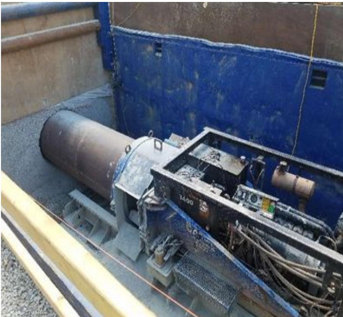
Fig 27: Midwest Mole Inc. continues to drill through ledge underneath Main St. Viewing southwest. (6-26-19).
