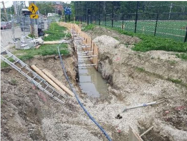
Fig 19: McCourt pumping residual water out of current work area, into existing Trench along Colovos Rd. Viewing south. (6-25-19).
