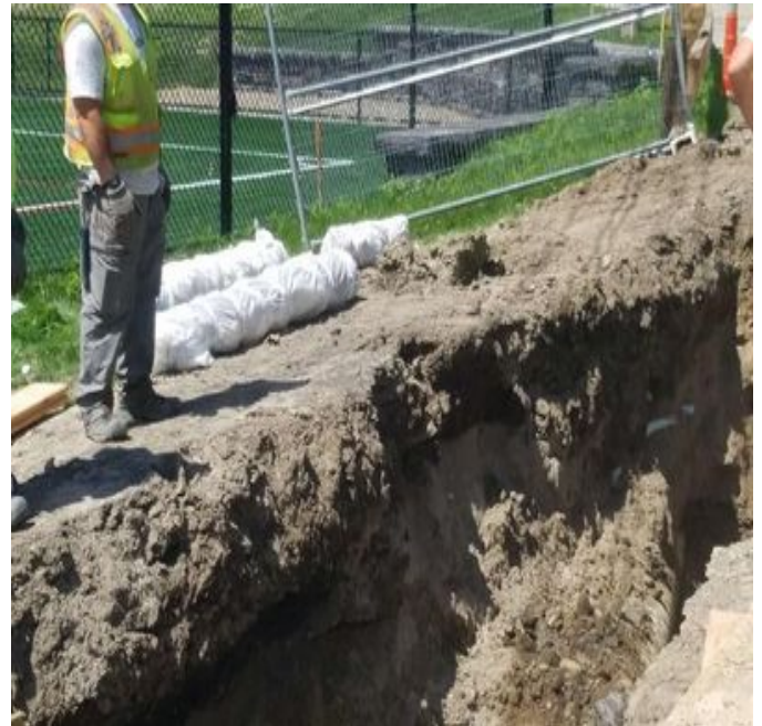
Fig 16: Asbestos pipe properly secured, waiting to be picked up. Viewing north. (6-24-19).
