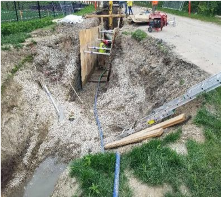
Fig 17: McCourt excavating next to Colovos Rd, north of existing trench, moving towards steam pipe. Viewing north. (6-25-19).
