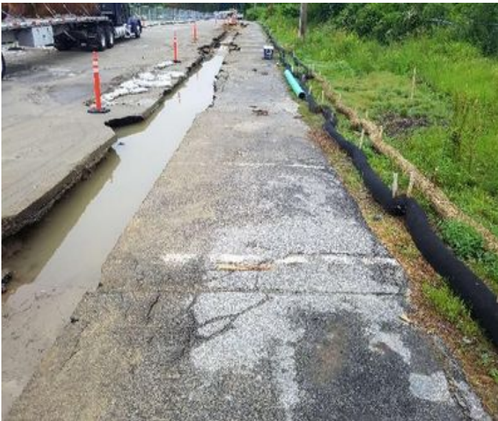
Fig 23: Silt sock installed next to trenching activities in "A" lot. Viewing north. (6-26-19).
