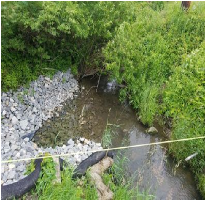
Fig 9: No sediment observed discharging into College Brook as a result of trench dewatering activities next to Colovos Rd. Viewing east. (6-21-19).
