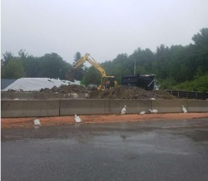
Fig 1: GZA continues to haul out soil from stockpile area in "A" lot. Viewing north. (6-20-19).
