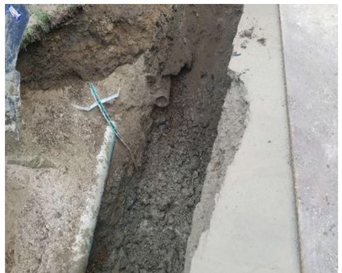
Fig 20: Residual water seeping out from stone beneath old water pipe. Viewing north. (6-25-19).
