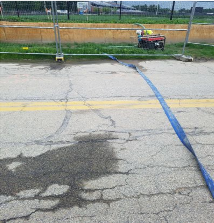
Fig 5: Test pump, 2in electric pump pumping rain water from trench. Viewing west. (6-21-19).
